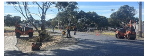
Above: Pavement construction works underway at Fulwood Avenue and Northcott Terrace, Tintinara.
